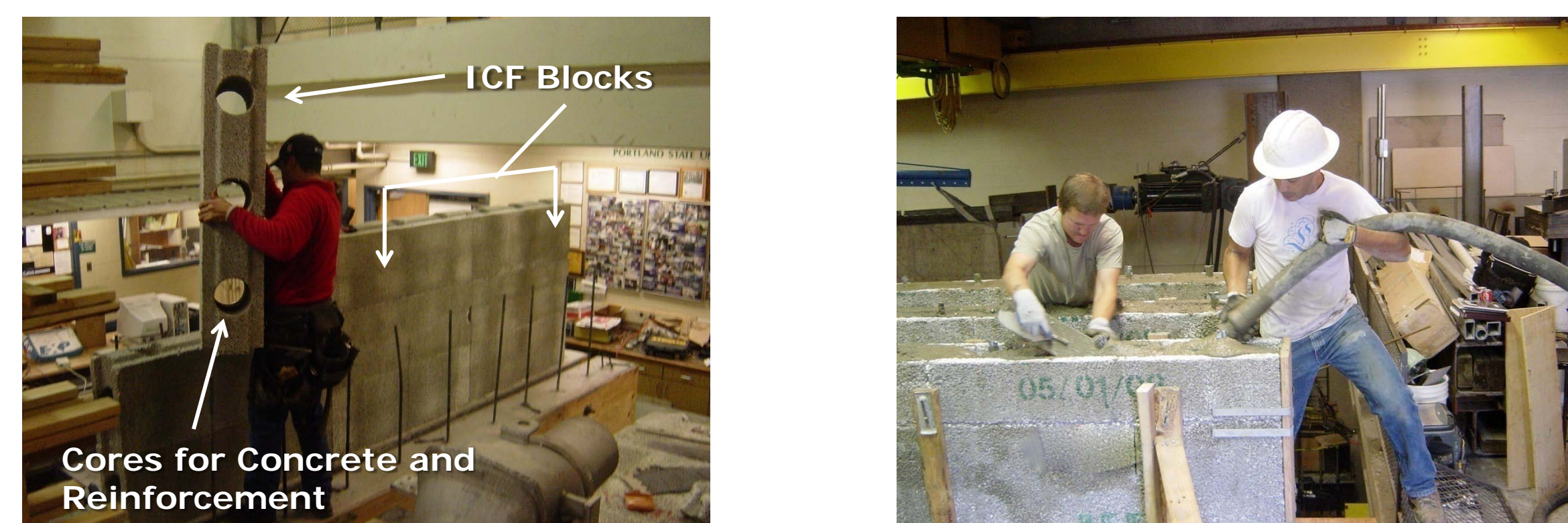
(A) Erection of ICF grid wall form (B) Concrete placement in cores
